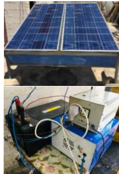
Figure (4): Electric Solar Components.
