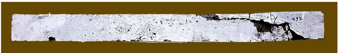
Plate 17 Crack pattern and mode of failure of bubbled slab (G5-S4)
