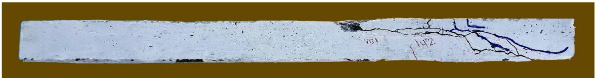
Plate 14 Crack pattern and mode of failure of bubbled slab (G5-S1)
