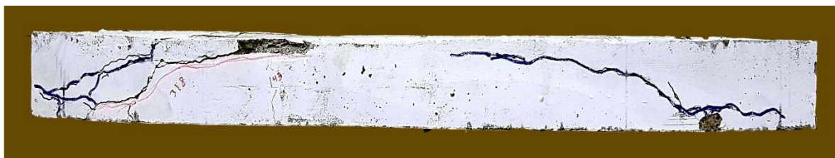
Plate 8 Crack pattern and mode of failure of bubbled slab (G3-S1)
