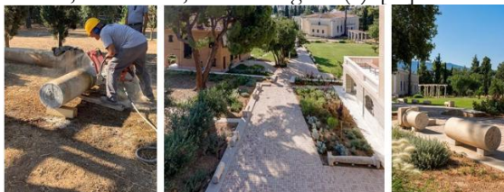
Figure (9): Ionic columns from the original entrance to the garden of the Greek Foundation for Culture and their reuse as benches and artistic paths in the garden (right, left, center) [40].
