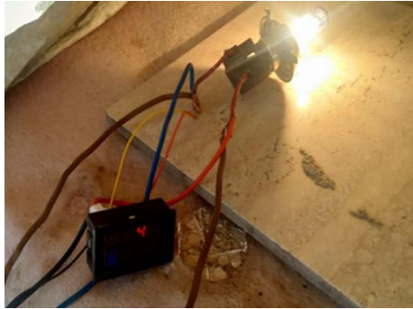
Figure (22): Mini Digital Voltage-Ampere meter and direct current electric lamp
