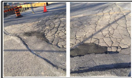
Picture (1): Fatigue cracking in flexible pavement [5]
